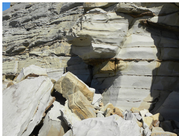
Fig. 1 Photograph of a fractured rock mass in Newcastle, NSW, Australia (photograph by O. Buzzi)
